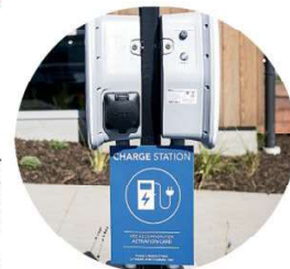
Charging stations are becoming more widespread.
